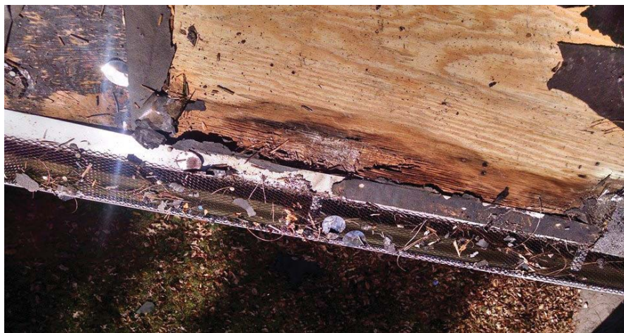
This roof deck has been damaged by repeated moisture intrusion due to ice dams. Photo courtesy of Air Vent.
