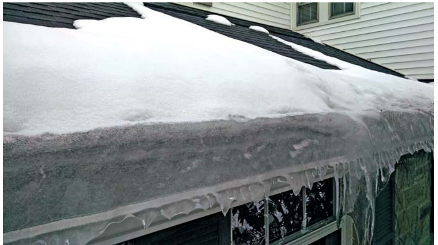
A classic ice dam—simply removing it will not solve the issue. Photo courtesy of Air Vent.
