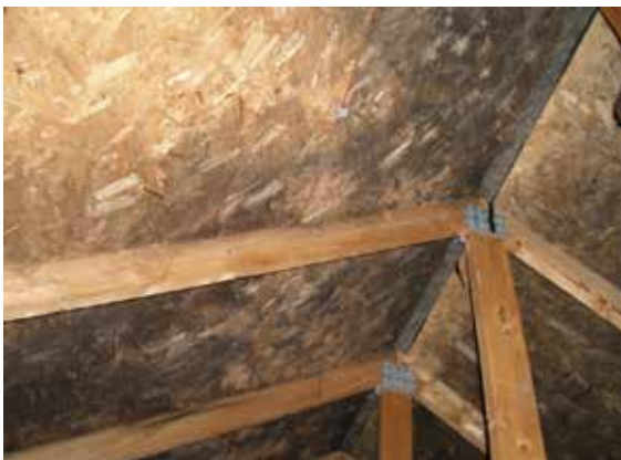
Note the discoloration under the decking,
