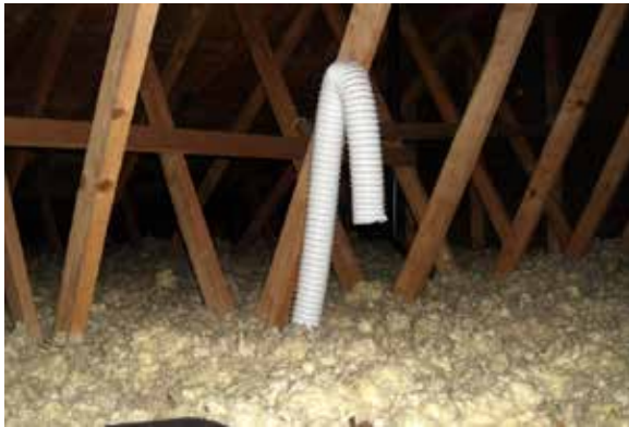
Excess moisture from improperly vented bathroom fans can result in mold growth.
