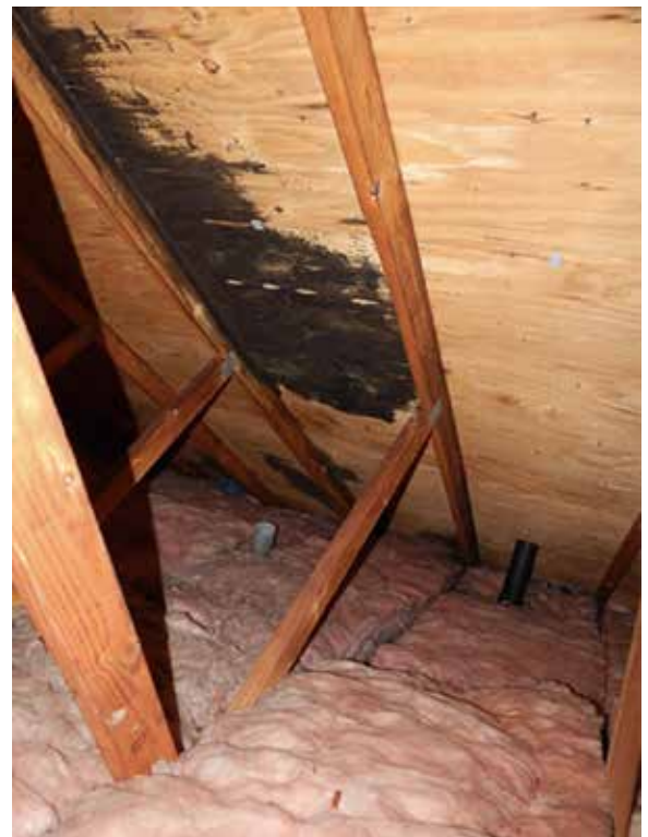
Excess moisture from improperly vented bathroom fans can result in mold growth.
