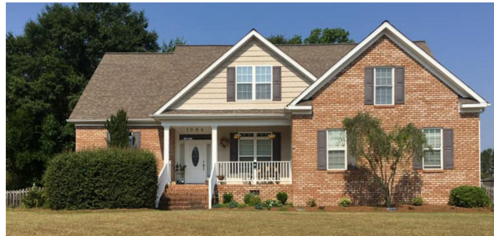
"We replaced all of the ridge vent and cap shingles on this home after replacing the OSB sheathing on both sides of the ridges. We reduced the opening size to Air Vent's recommended 3/4 inches on both sides of the ridge beam, instead of the nearly 4-inch gaps we found under the leaking ridge vents." – Trevor Atwell
