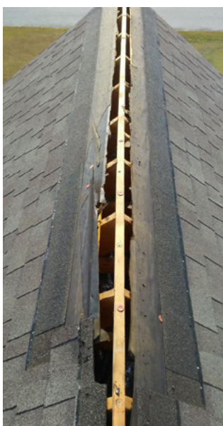
Nearly a 4-inch wide slot to the left of the ridge beam.
